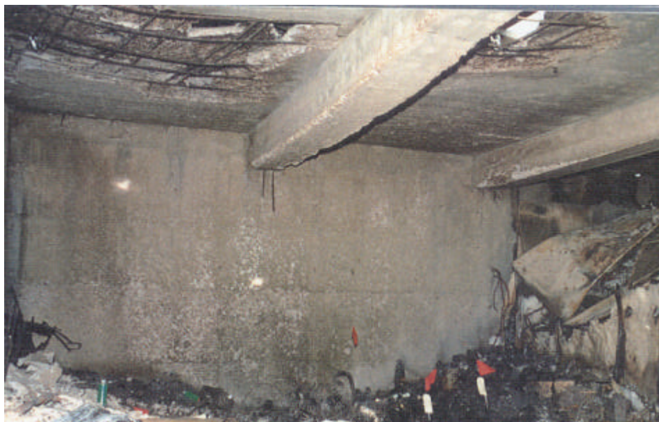
Figure 6.3 Spalling occurred at several places of the bunker slab due to intense fire exposure from below and from above.
