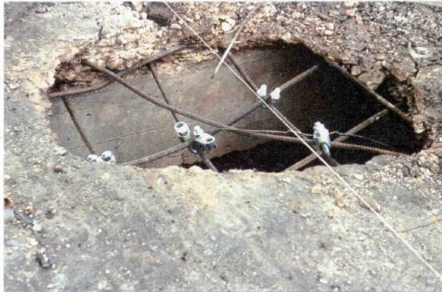
Figure 6.1 FBI photo. The hole in the concrete ceiling slab of the bunker. Note the poor concrete quality.
