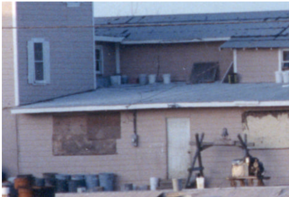
Figure 3.5 FBI ground photo from the Black Side of the cafeteria. The board covering of the window to the left of the door appears weak and may have fallen when liquid fuel was ignited and the interior pressure increased.
